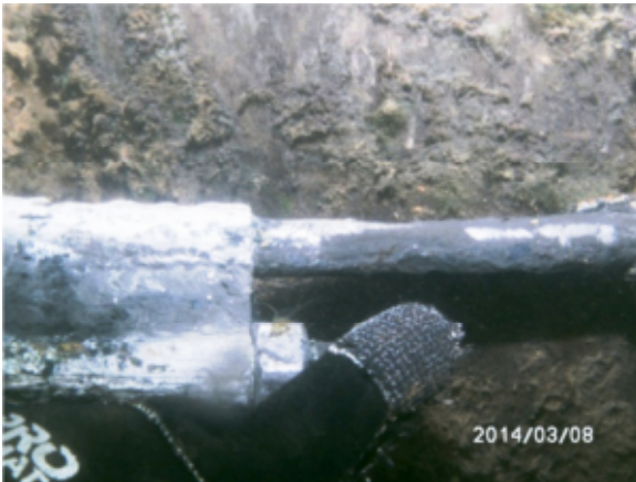
Photo 21A – Stripped / corroded connector
