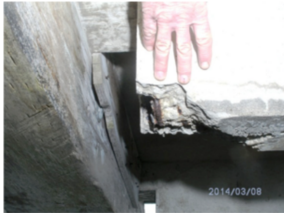
Photo 16A – Spalling at underside of precast "T"
