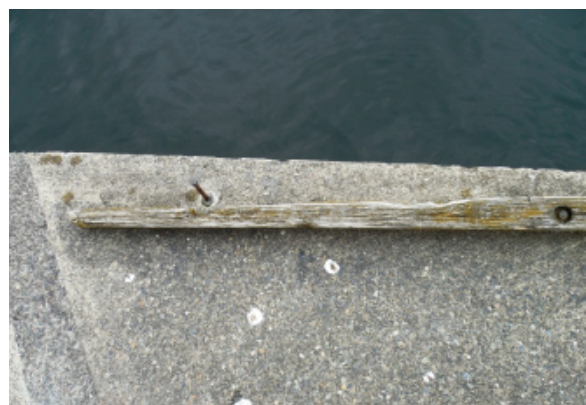
Photo 12A – Deteriorated / loose bull rail
