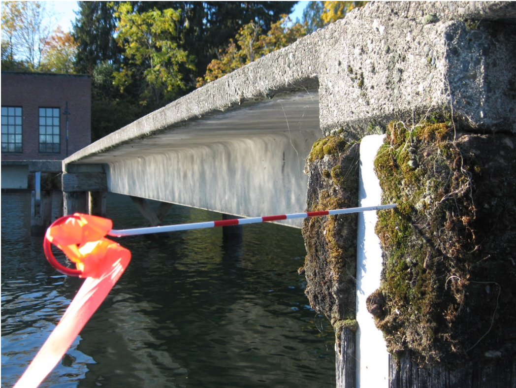
Figure 2: Detail of cap beam illustrating typical rot condition
