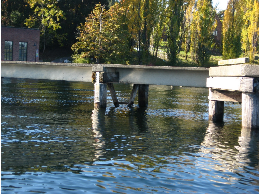
Figure 1: Profile view of pier showing concrete panel and wood cap beam construction
